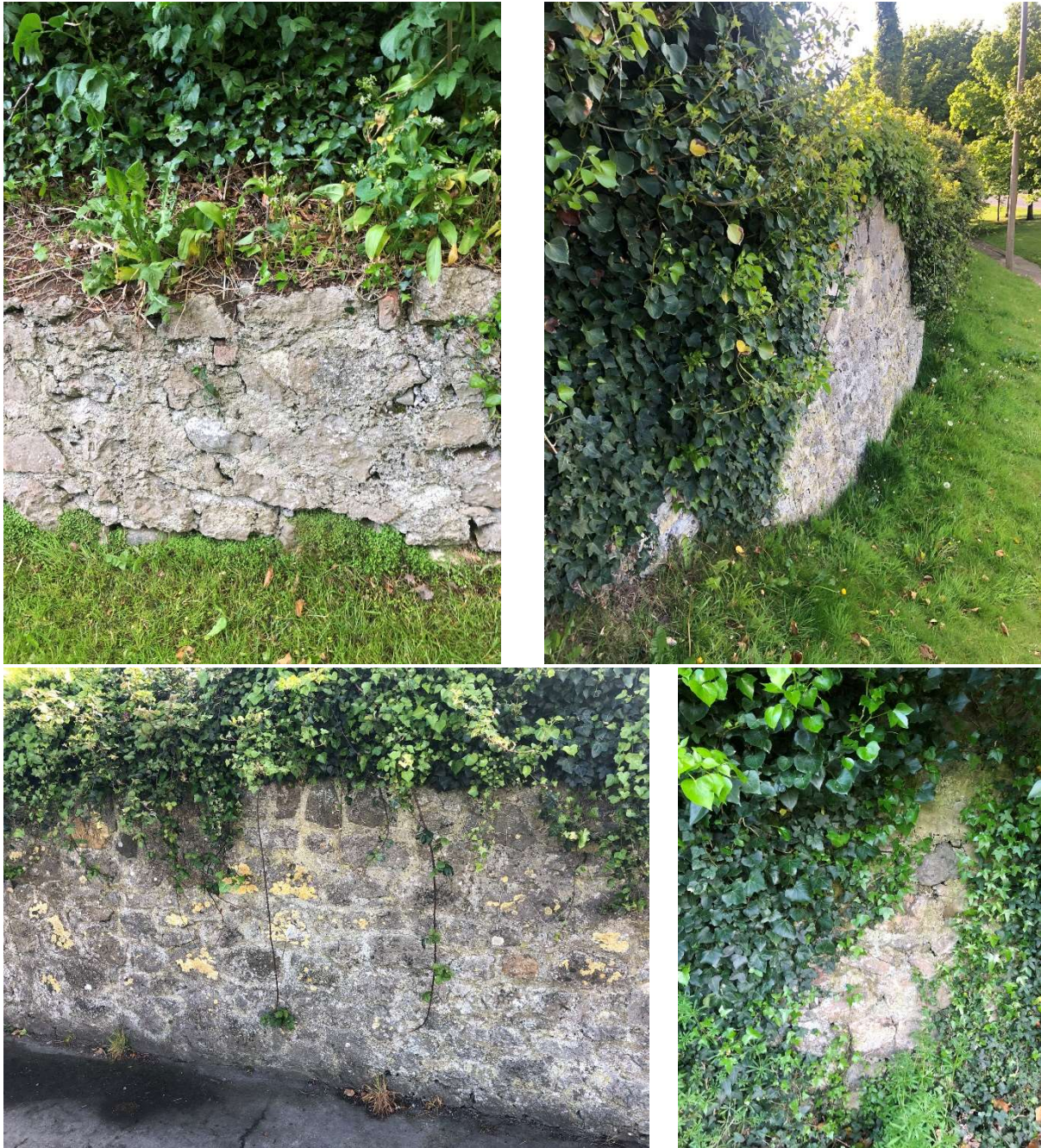
Figure 15.8: Photographs along the historic boundary wall to the northern and eastern boundaries of the subject site
